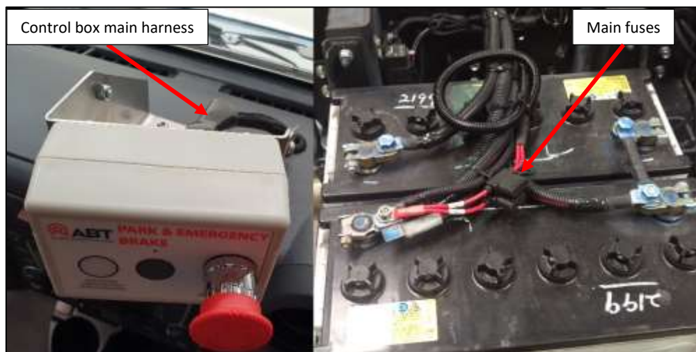
Fig 5: Failsafe EM control box and power connections.
