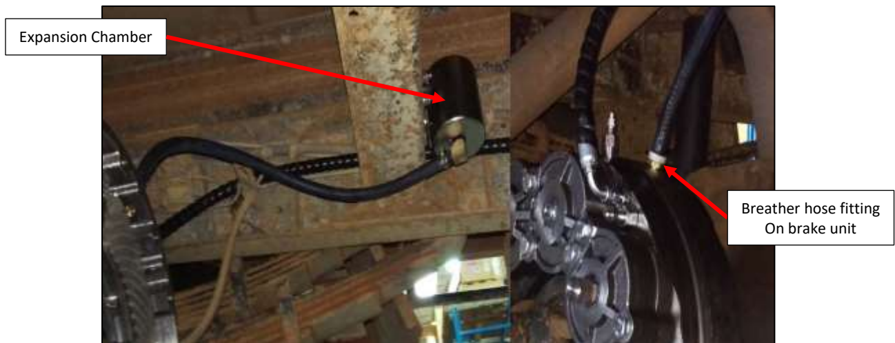
Figure 4: Brake Expansion Chamber and breather hose.
