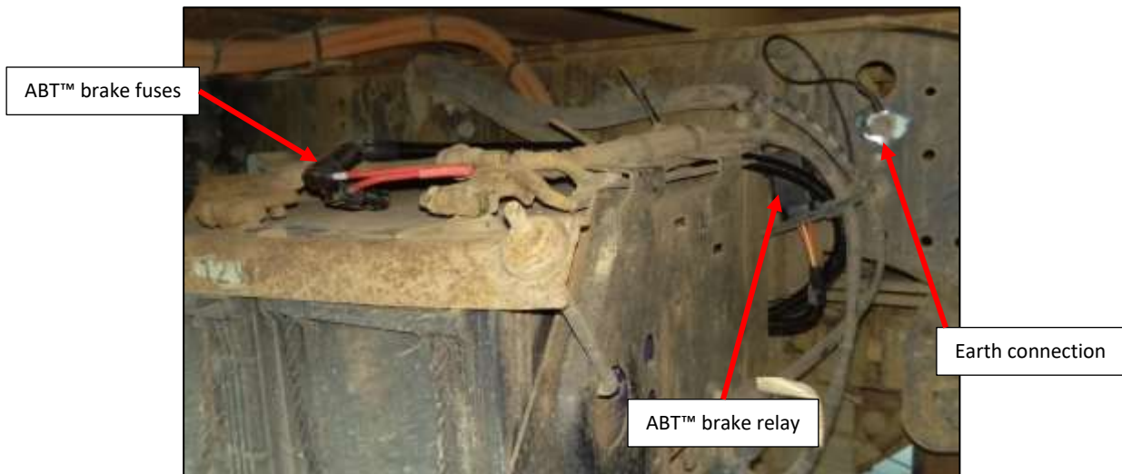
Figure 14: Battery power harness.
